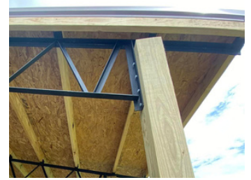
Bar Joist Steel Trusses
