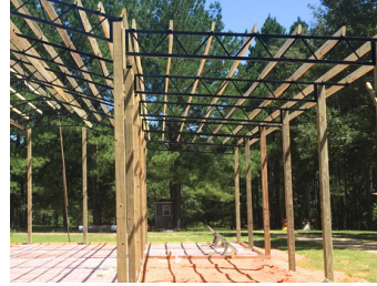
Lean-To Steel Trusses
